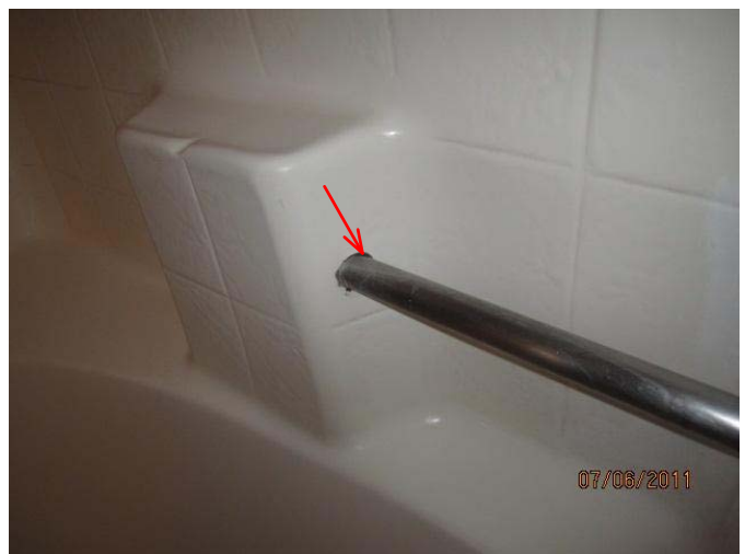
#54 Shower grab bar needs to be sealed
