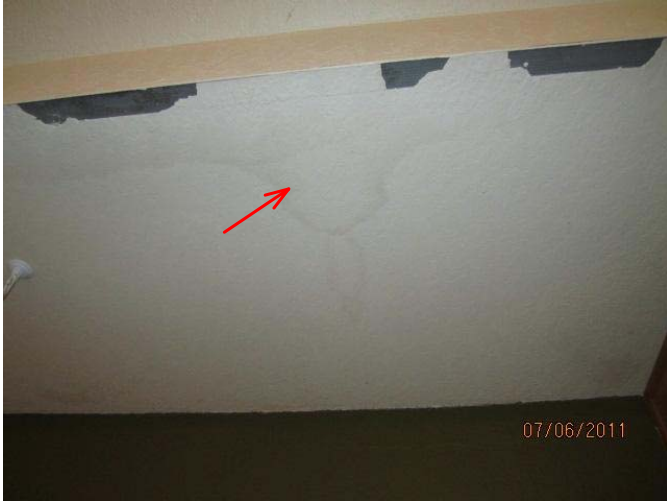
#73 Moisture stains noted to ceiling, suspect its from a roof leak
