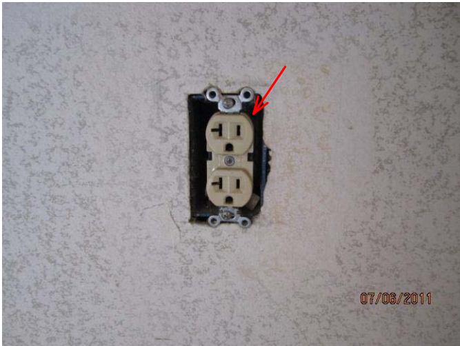
#33 Missing outlet cover plate at laundry area
