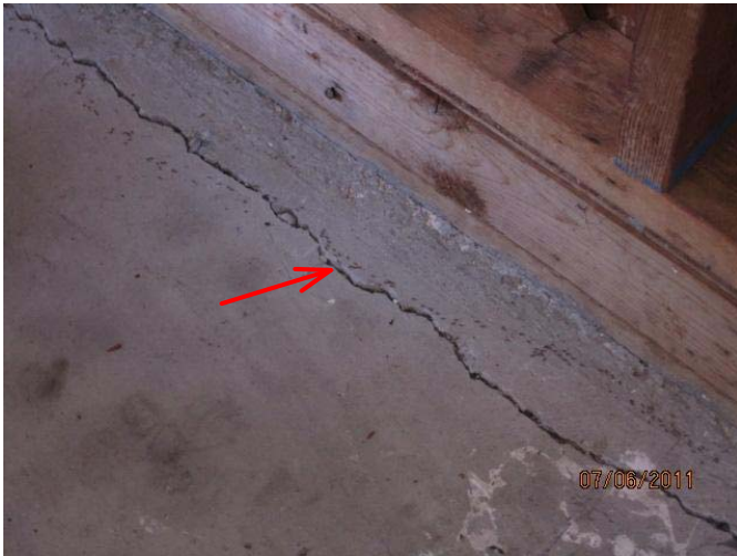
#27 Garage floor cracks noted
