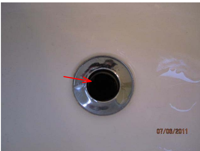
#47 Sink stoppers are missing
