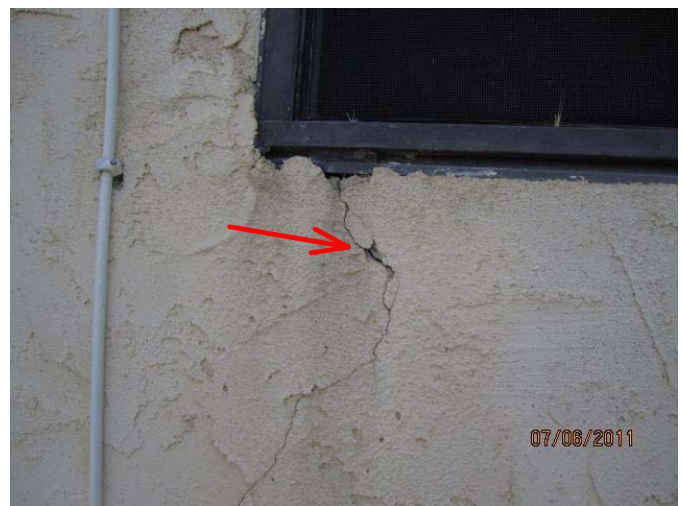
#18 Stucco cracks need repair
