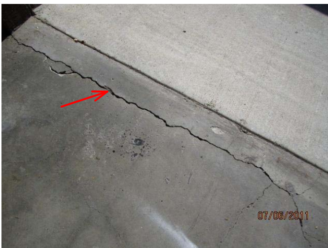
#29 Garage floor cracks noted
