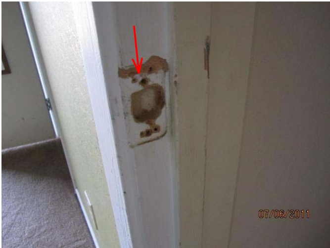
#45 Missing door hardware
