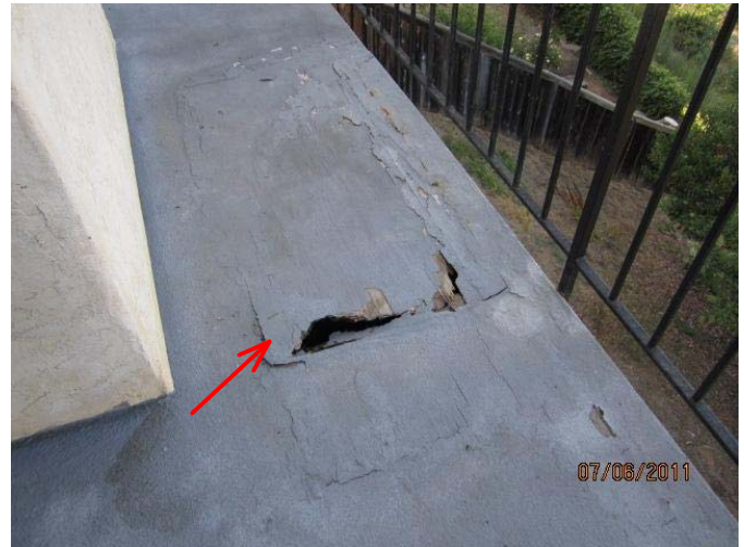
#82 Balcony has extensive rot and is not safe to walk on
