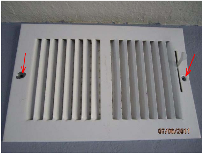
#61 Vent covers are not secured
