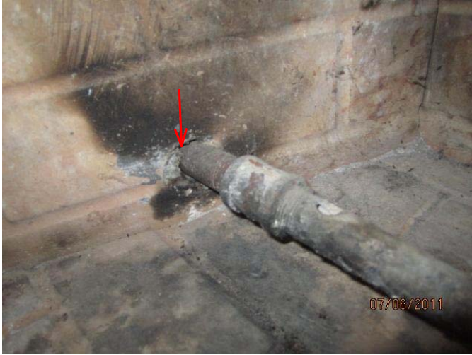
#79 Gas port needs to be re-sealed
