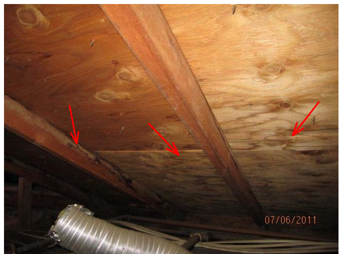
#90 Excess moisture stains noted
