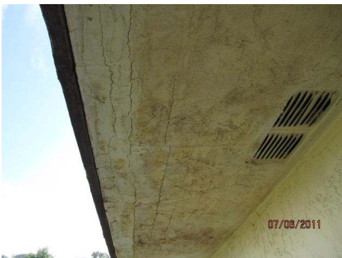
#83 Moisture damage to under side of upper deck due to wood rot
