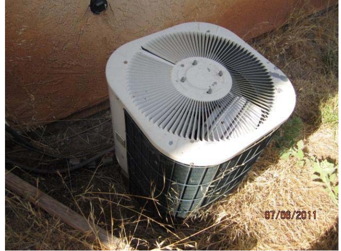
#14 AC unit should be lifted off the ground to allow water to drain under the unit
