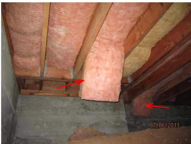
#65 Loose insulation needs to be secured
