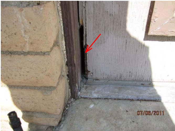
#9 Garage door has wood rot
