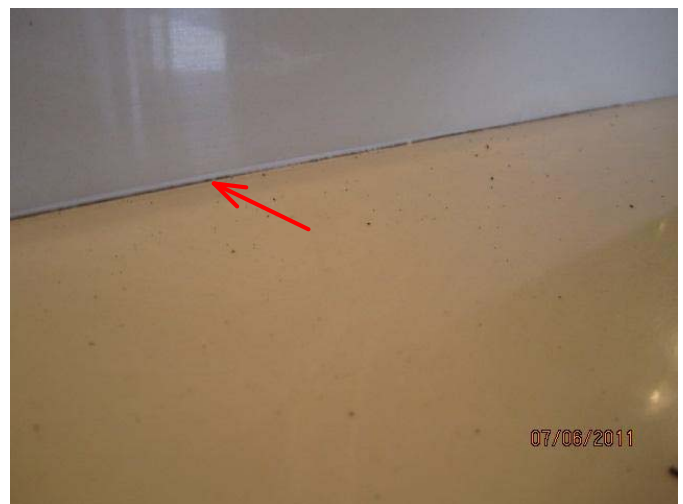
#48 Counter tops need to be re-sealed
