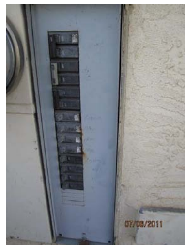
#24 Main Electrical Panel cover hinges need repair
