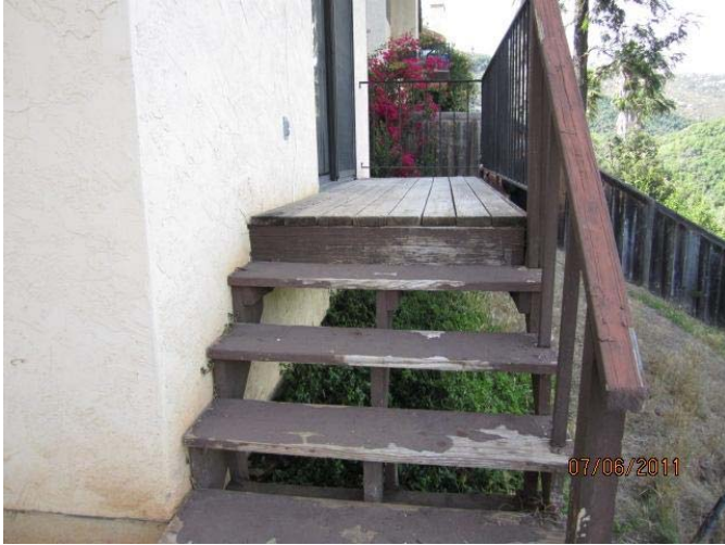
#19 Wood deck should be re-built due to wood rot
