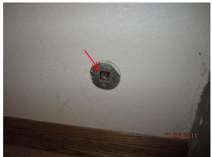
#78 Gas valve key is missing
