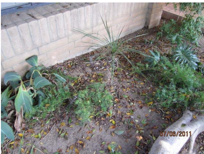
#5 No drainage located at front of house, recommend improving grading
