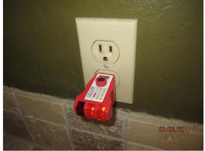
#68 No GFI in kitchen
