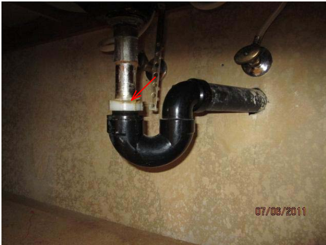
#87 Drain pipe connection is cracked
