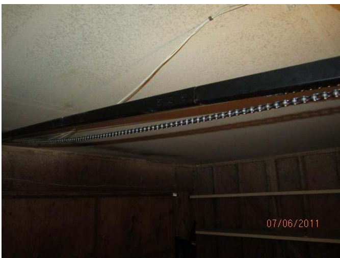
#41 Garage door opener needs adjustment
