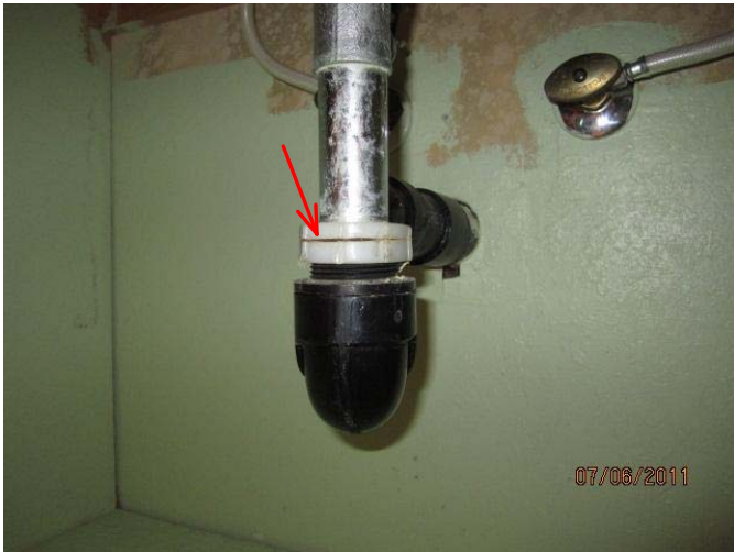
#57 Sink drain pipe connection is cracked
