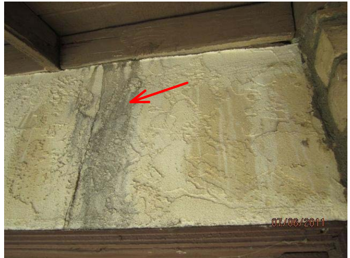
#10 Water stains indicate the roof may be leaking
