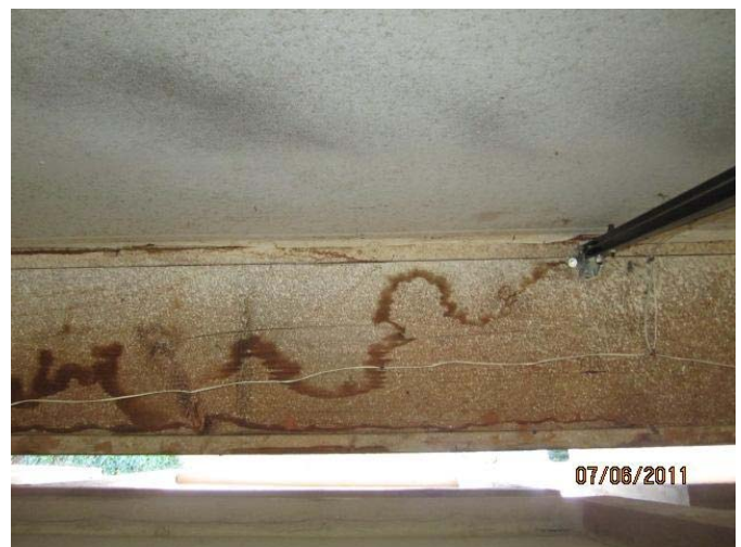
#30 Stains above garage door, suspect a roof leak
