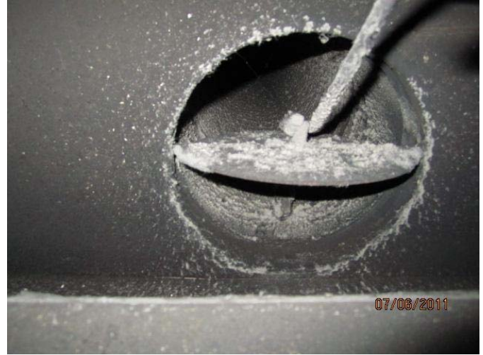
#80 Creosote build-up, recommend cleaning
