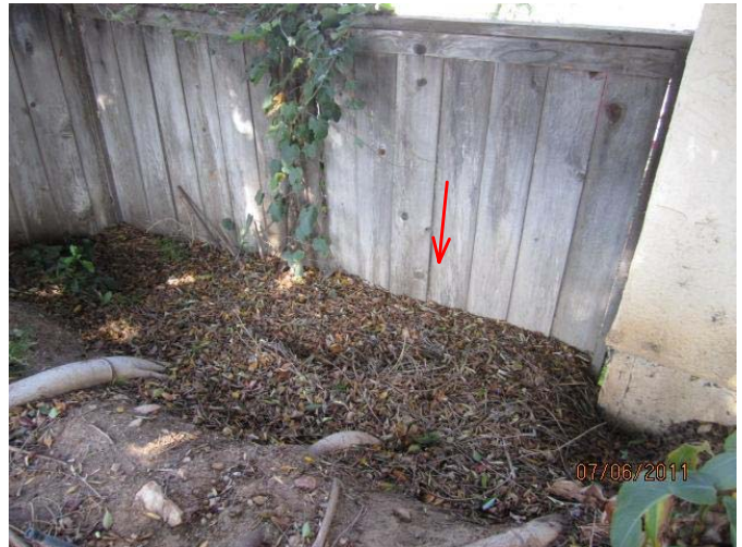
#4 Wood fence is rotting due to poor drainage
