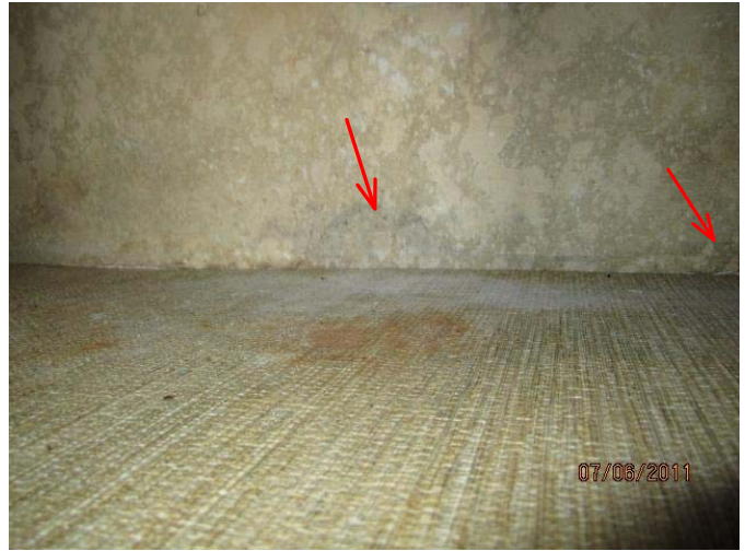
#50 Moisture stains noted under sink, suspect possible mold
