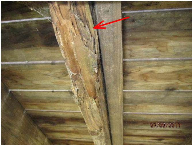
#21 Wood deck should be re-built due to wood rot
