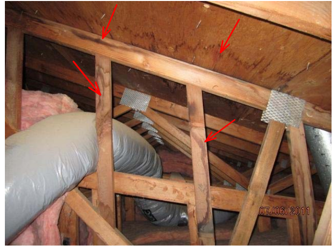
#92 Excess moisture stains noted
