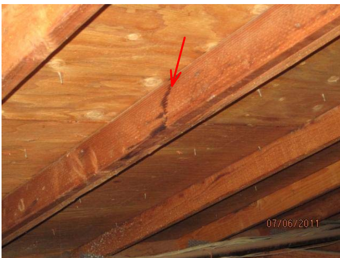
#89 Excess moisture stains noted
