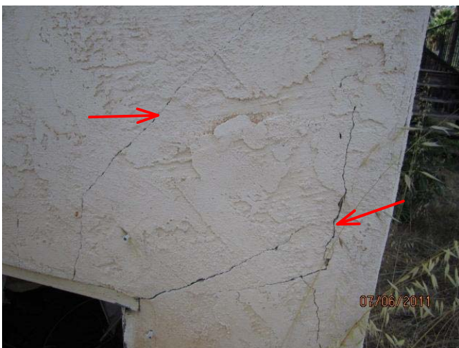
#23 Stucco cracks need repair
