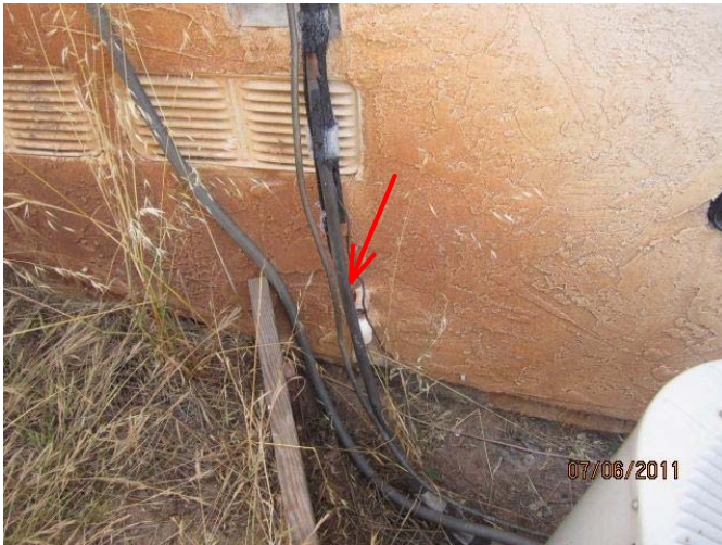
#15 AC line insulation needs to be replaced
