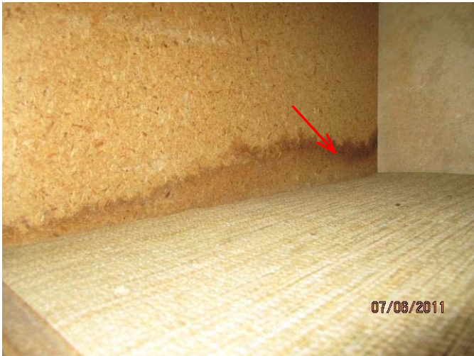
#51 Moisture stains noted under sink
