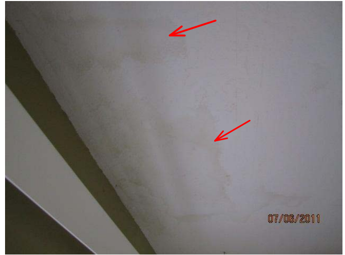
#44 Moisture stains noted, suspect it's from the deck leak
