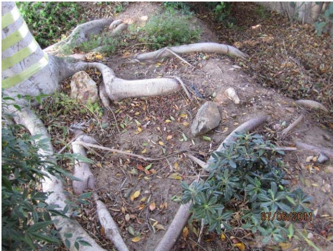
#3 Tree roots can cause foundation problems
