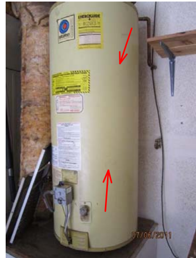
#34 Hot water heater is missing straps
