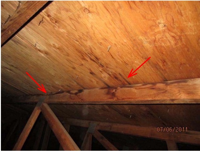
#91 Excess moisture stains noted
