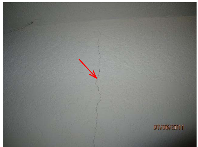
#60 Drywall cracks noted
