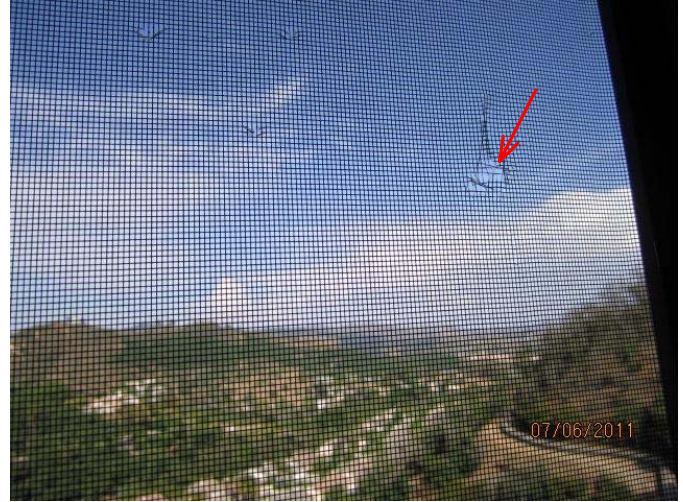
#74 Torn window screens
