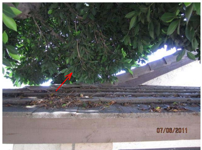
#6 Trees should be cut back from the roof
