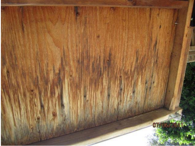
#31 Garage door has water damage
