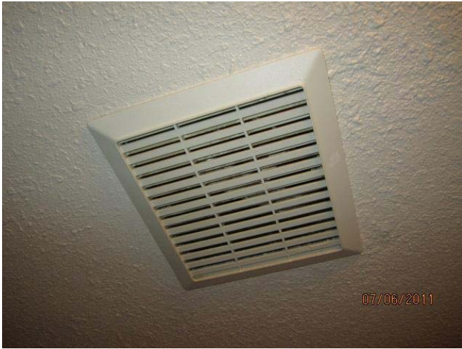
#55 Electric vent fan does not work
