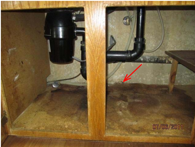
#69 Moisture damage, mold like substance noted under kitchen sink
