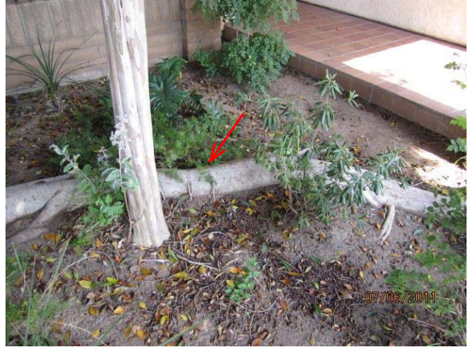
#2 Tree roots can cause foundation problems
