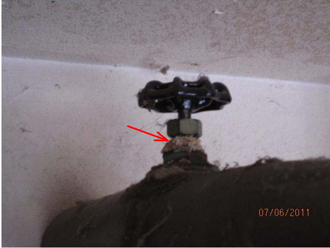
#37 Tank isolation valve needs to be replaced
