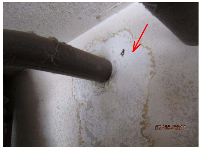
#36 Water stains, suspect a past leak as it's currently dry
