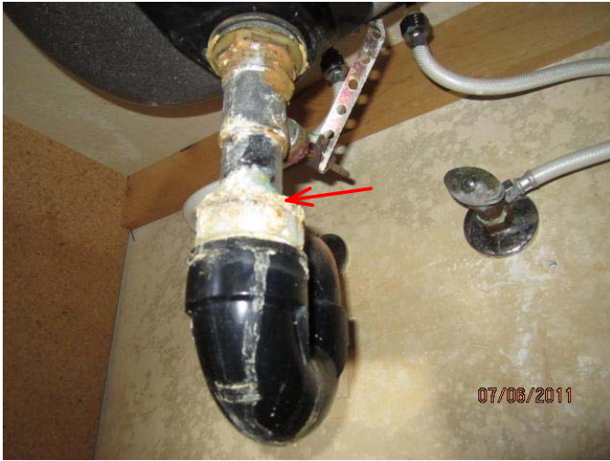
#49 Sink drain connection is corroded and cracked
