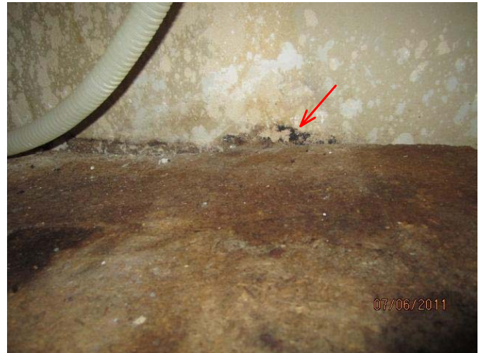
#70 Mold like substance noted under kitchen sink
