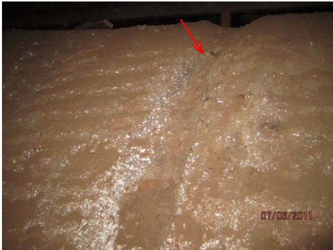
#63 Signs of water intrusion from the front foundation wall
