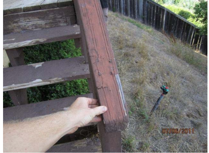
#20 Wood deck should be re-built due to wood rot
