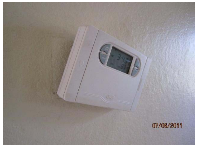
#42 Thermostat is loose
