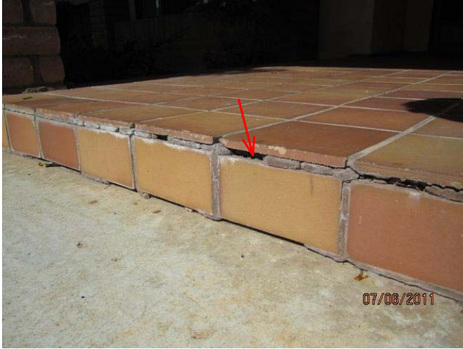
#7 Entry tile grout needs repair
