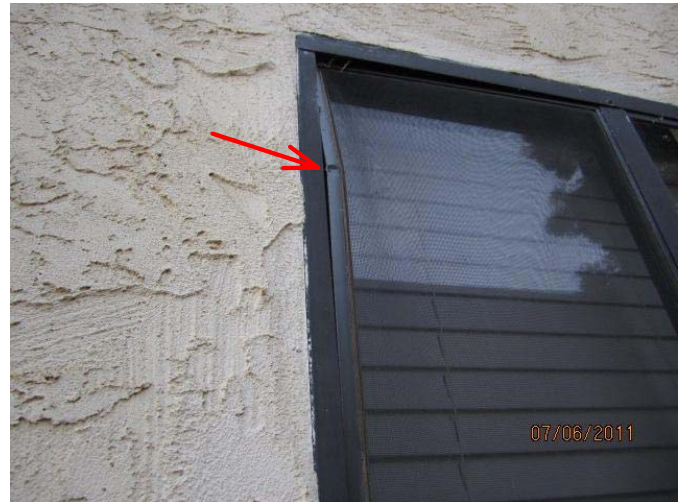
#22 Window screens are damaged
