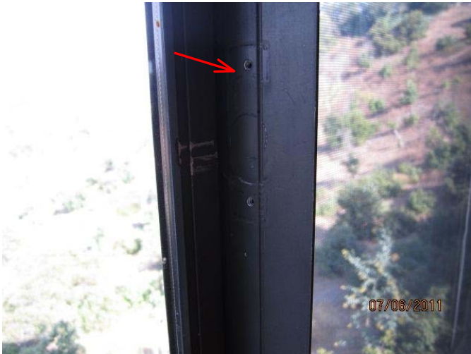
#75 Missing window hardware
