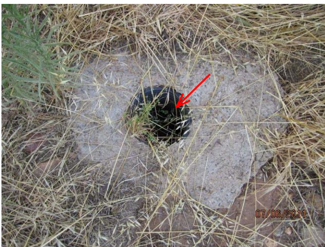
#17 Surface drains need covers
