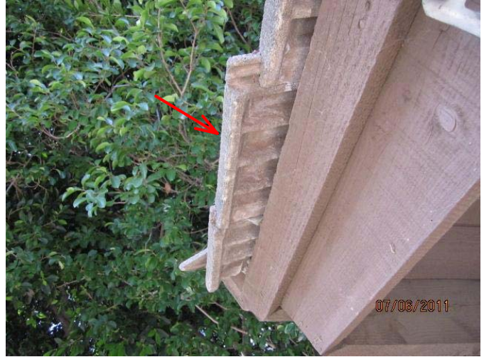
#8 Roof tiles have slipped
