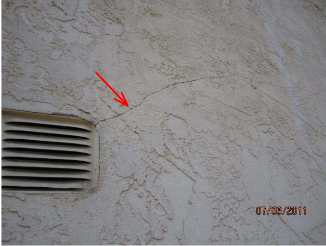
#13 Stucco cracks need repair
