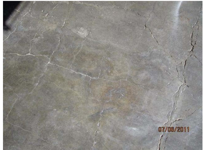
#28 Garage floor cracks noted
