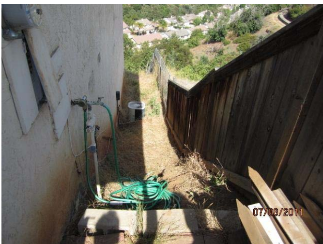
#11 Side yard needs steps and proper drainage
